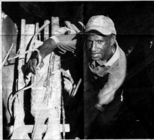
Rasa Communication worker Peter Gend attending to the burnt cable along Waigani Drive yesterday. Rasa Communication is contracted by Telikom to maintain affected lines. Nationalistic by EKAN KEAPO.
